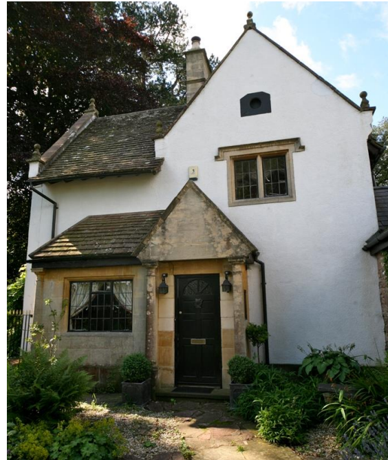
Fig.25 The Lodge to Shirenewton Hall rendered and painted white with ashlar dressings
